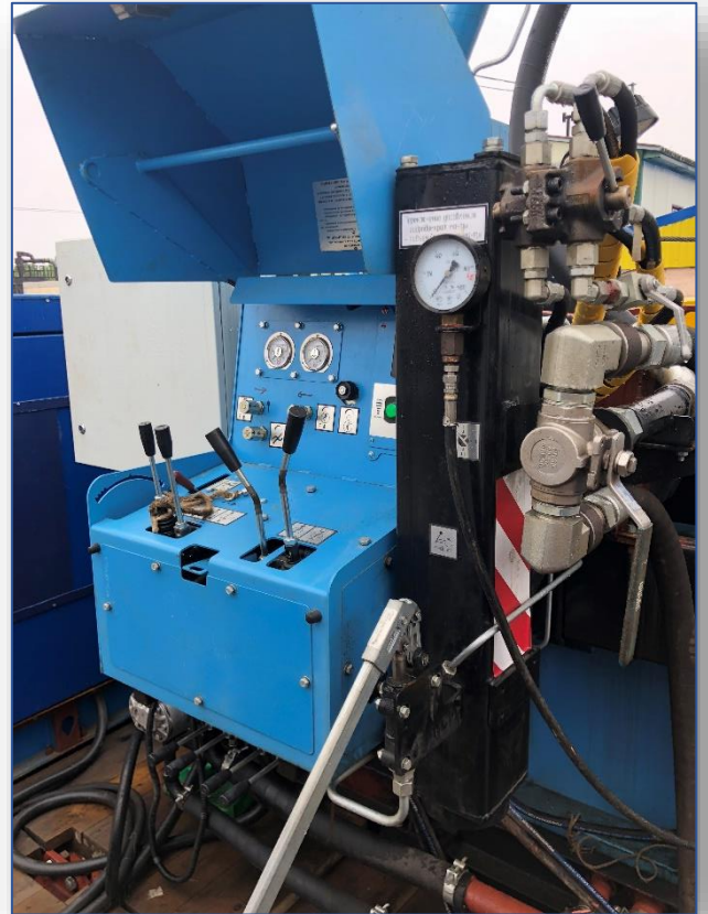
Drilling rig control panel
